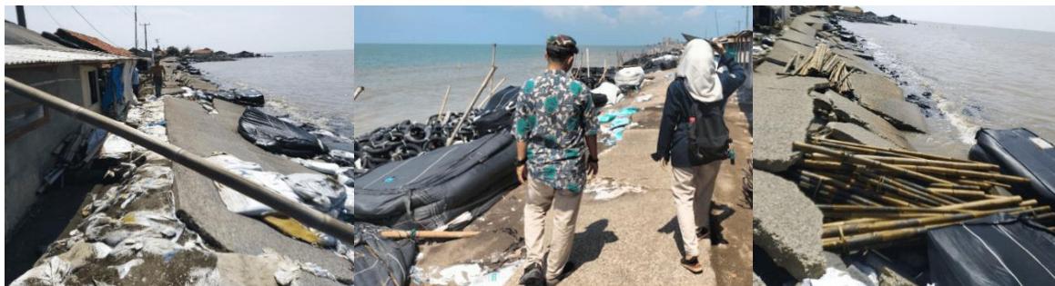
Figure 1. The condition of the access road was cut off due to abrasion (May 7, 2023)
